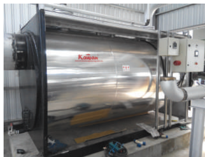
Hot water boiler for CTI test facility
