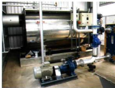
Hot water boiler for CTI test facility
