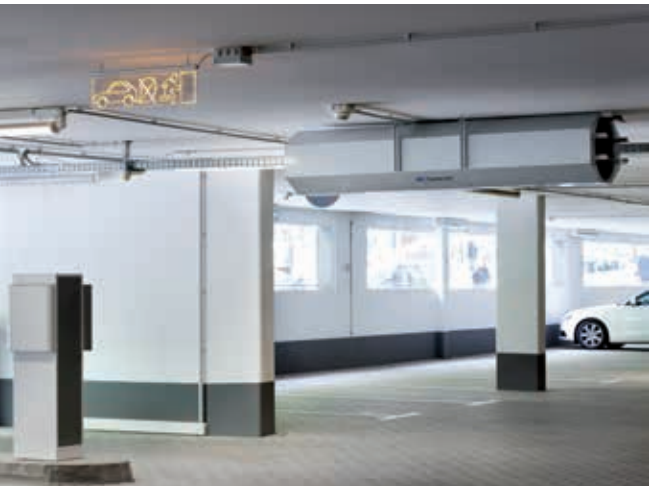
Installed premium jet fan
