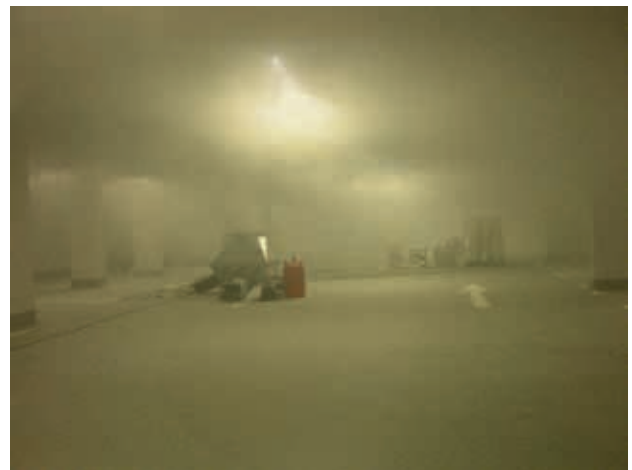
Smoke gas test during commissioning
