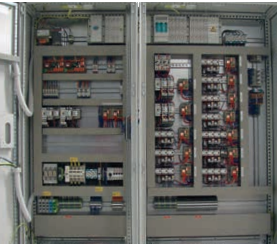
Control cabinet with control modules
