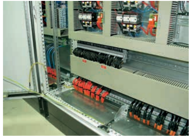
Installed supply cable for Jets and main fans
